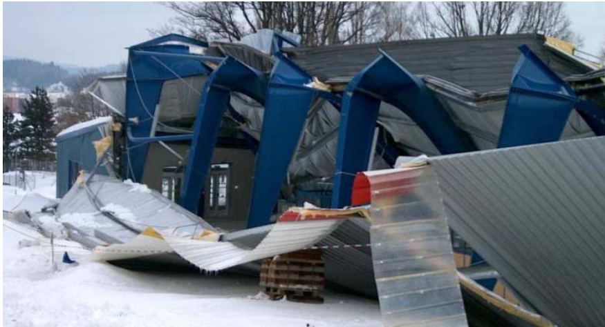
Figure 2. Collapse of a stadium.
