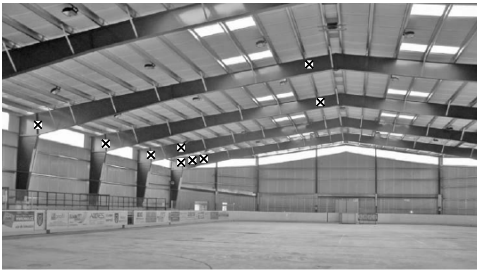
c) missing lateral buckling struts
