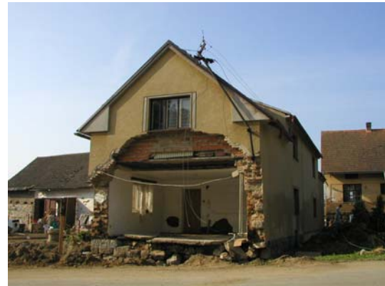
b) missing ring beams
