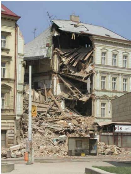
a) undermined foundations
