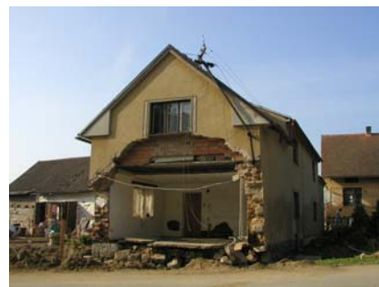
b) missing ring beams
