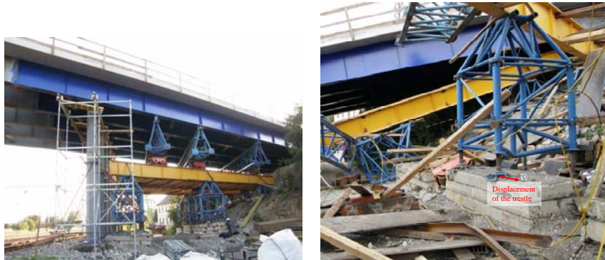
a) the bridge before collapse
